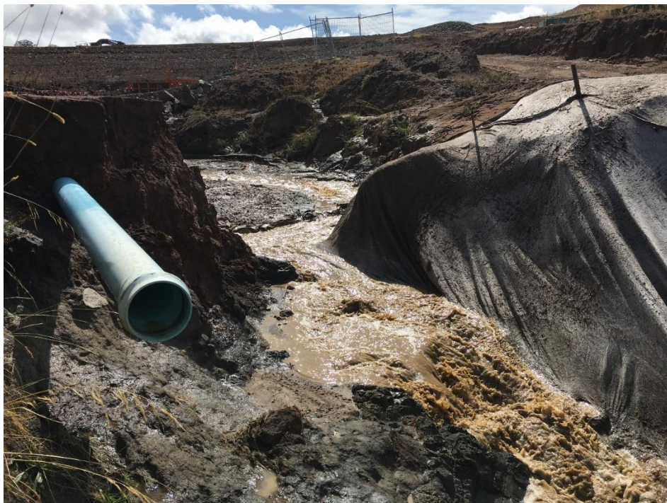
Figure 18. Failure of the Deep Creek sediment detention pond wall, February 2020. Source: ACT Waterwatch.
