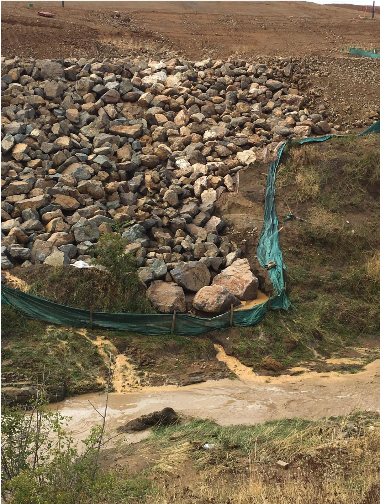
Figure 16. Sediment entering Deep Creek from construction areas, illustrating the failure of silt fencing to contain the mobilized sediment, February 2020. Source: ACT Waterwatch.
