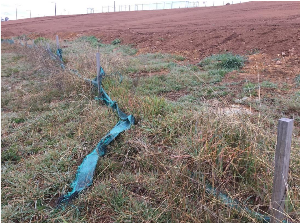
Figure 20. Poorly maintained silt fencing associated with urban development in the ACT. Source: ACT Waterwatch.
